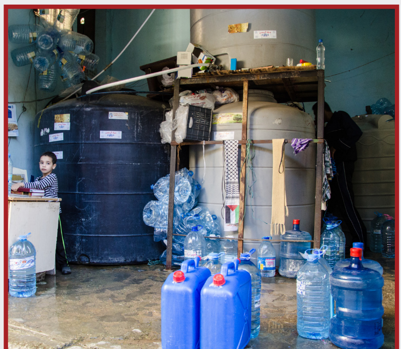
Water Purification Facility inside the Camp
